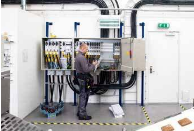
Distribution board in powder coated enclosure mounted on the wall in a switchgear room at a bakery, in Gothenburg, Sweden.
