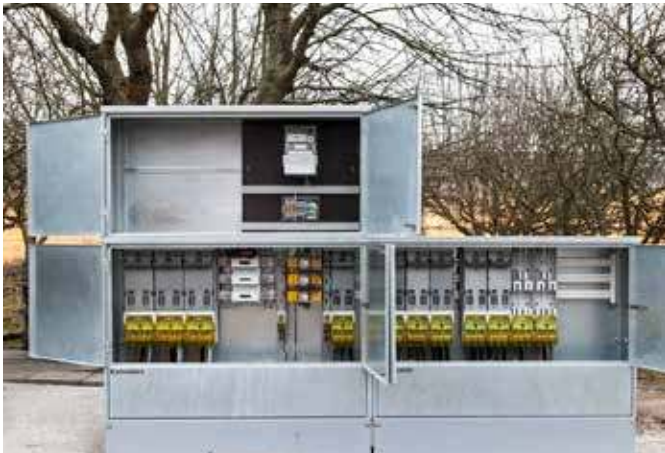
Cable distribution board, Sweden.
