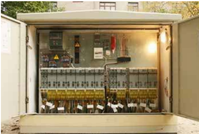
Kabeldon switching devices in a CSS, Latvia.
